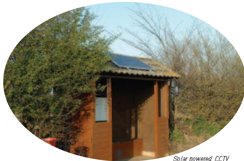
Solar powered CCTV
