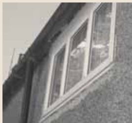
Poor quality imitation sliding sash UPVC windows
