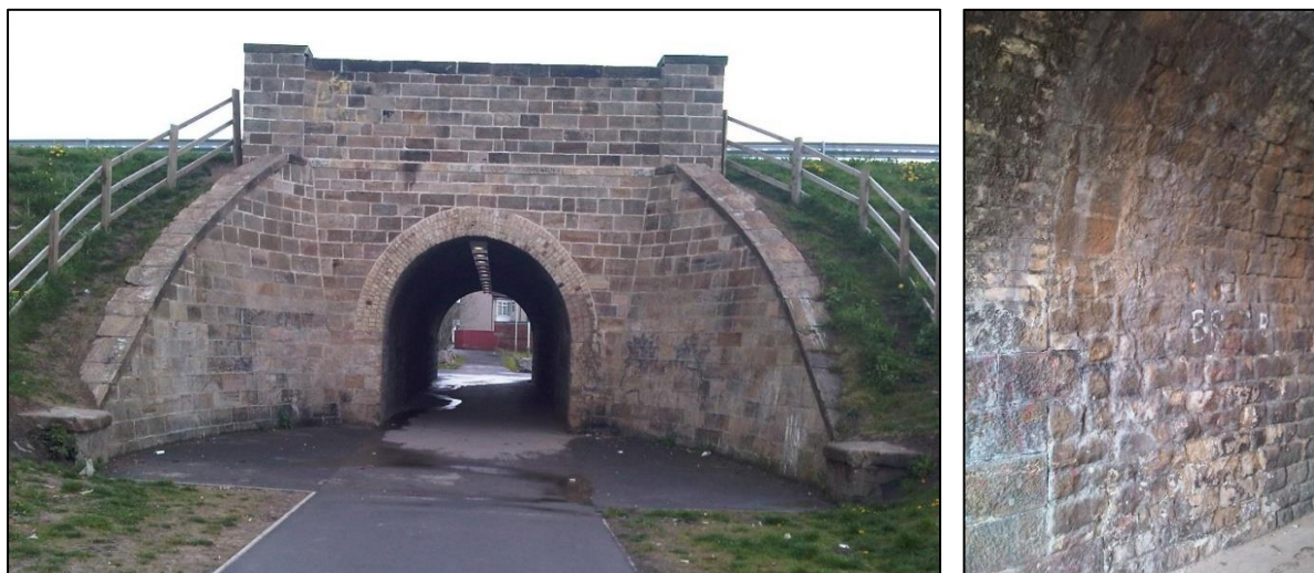
Plate 19. The extended accommodation bridge at Haughton Road and the distinct line inside showing where it was extended, also known as the Arnold Road Subway.
