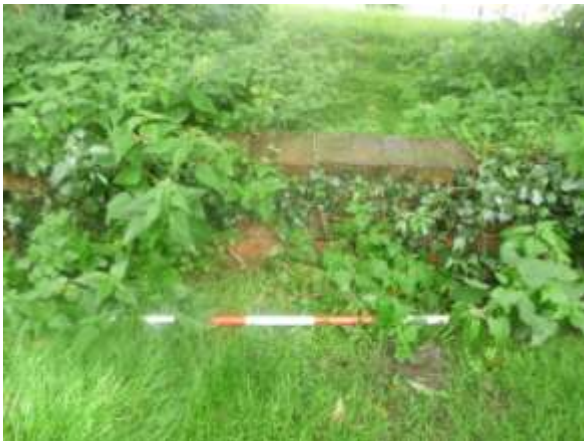
Plate 5. Part of the ha-ha south of the house, now leaning southwards and in need of maintenance
